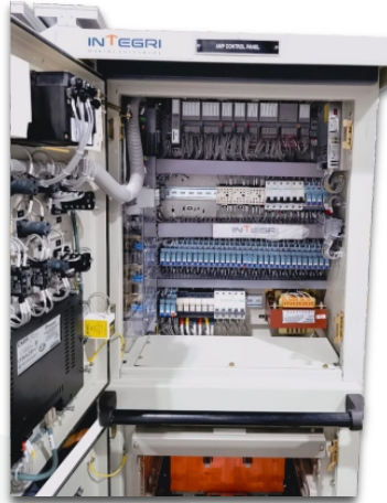
AMP/OPS Control Panel
