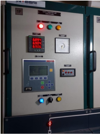
Supply from on shore power
